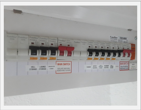
DB-2 Heating Location: Hallway
