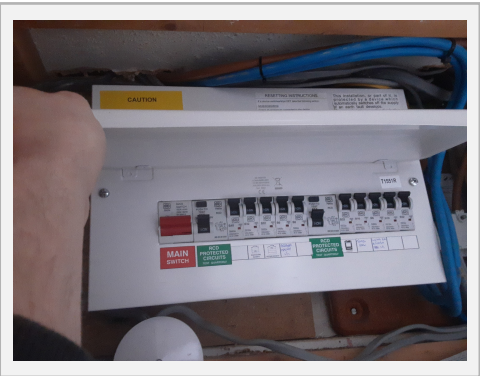
DB-1 Domestic Location: Hallway Cupboard
